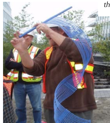
New hydronic radiant "capillary mat" system (pictured left) imported from Germany used on some of the buildings for radiant heating
